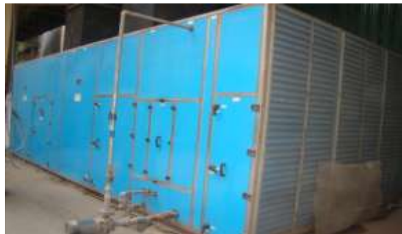
Cold fresh air ventilation system
